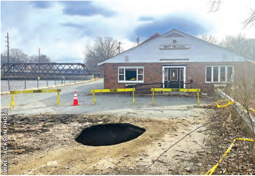
On Wednesday a sinkhole opened up in Turners Falls in the parking lot at 42 Canal Street, just next to the White Bridge to Greenfield. This newspaper received many reports of the hole. As of 4:30 p.m. it was surrounded by sawhorses belonging to the public works department and continuing to actively crumble. "It's on private property," public works superintendent Sam Urkiel told us when reached for comment. "The property owner should be contacted." Curt Sherrer, who has been renovating the property into a cidery and restaurant since 2018 and owns it under a trust, did not respond to a request for comment as of press time.
