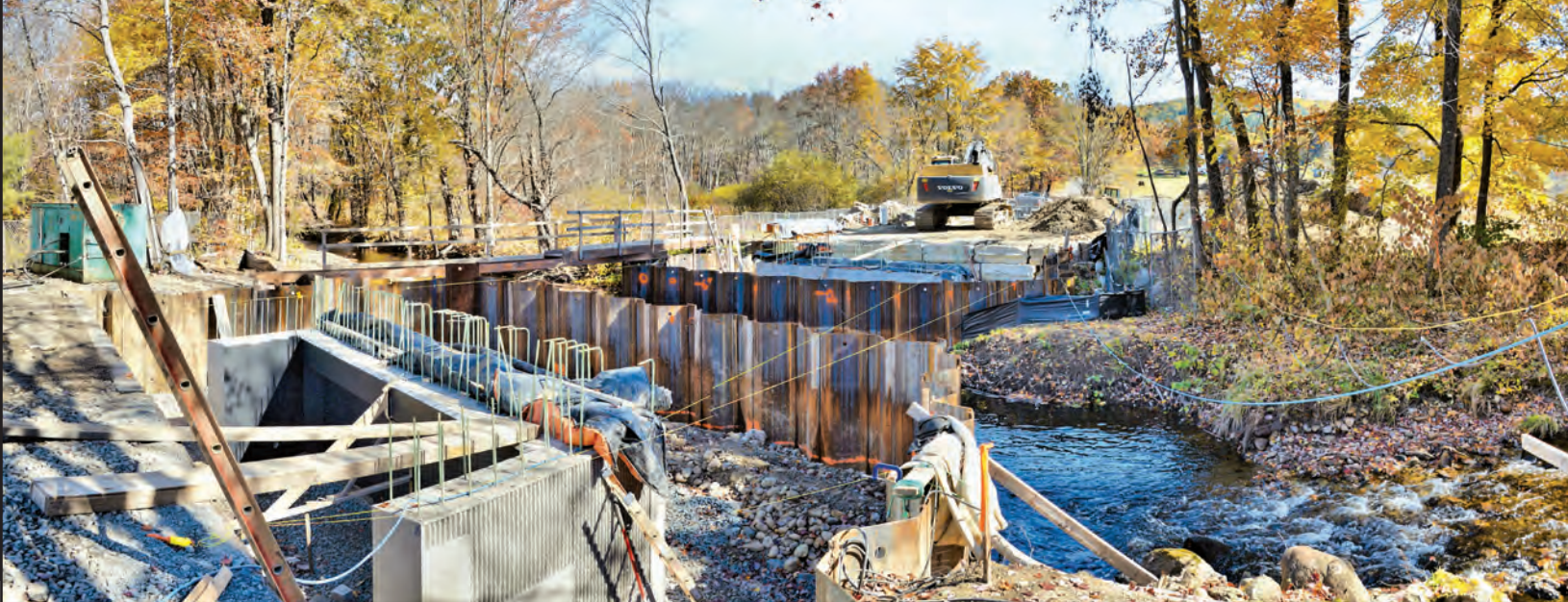
“Bridgework spanning the Sawmill River at Montague Center is beginning to take shape,” photographer Ed Gregory reports. “We’re at the southeast corner of the project, looking north. [At] lower left is the basal abutment for the south portal of the new bridge. Heavy steel sheeting driven deep into the earth maintains dry work areas on both sides of the river as it casually meanders 2.5 miles southwesterly to its confluence with the Connecticut River.” This photo was taken on Sunday.
