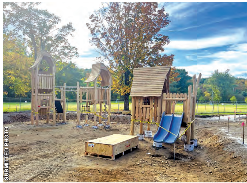
The Montague Center playground improvement project is well under way. Parks and rec director Jon Dobosz sent in this photo last week of the newly-installed play structures.
