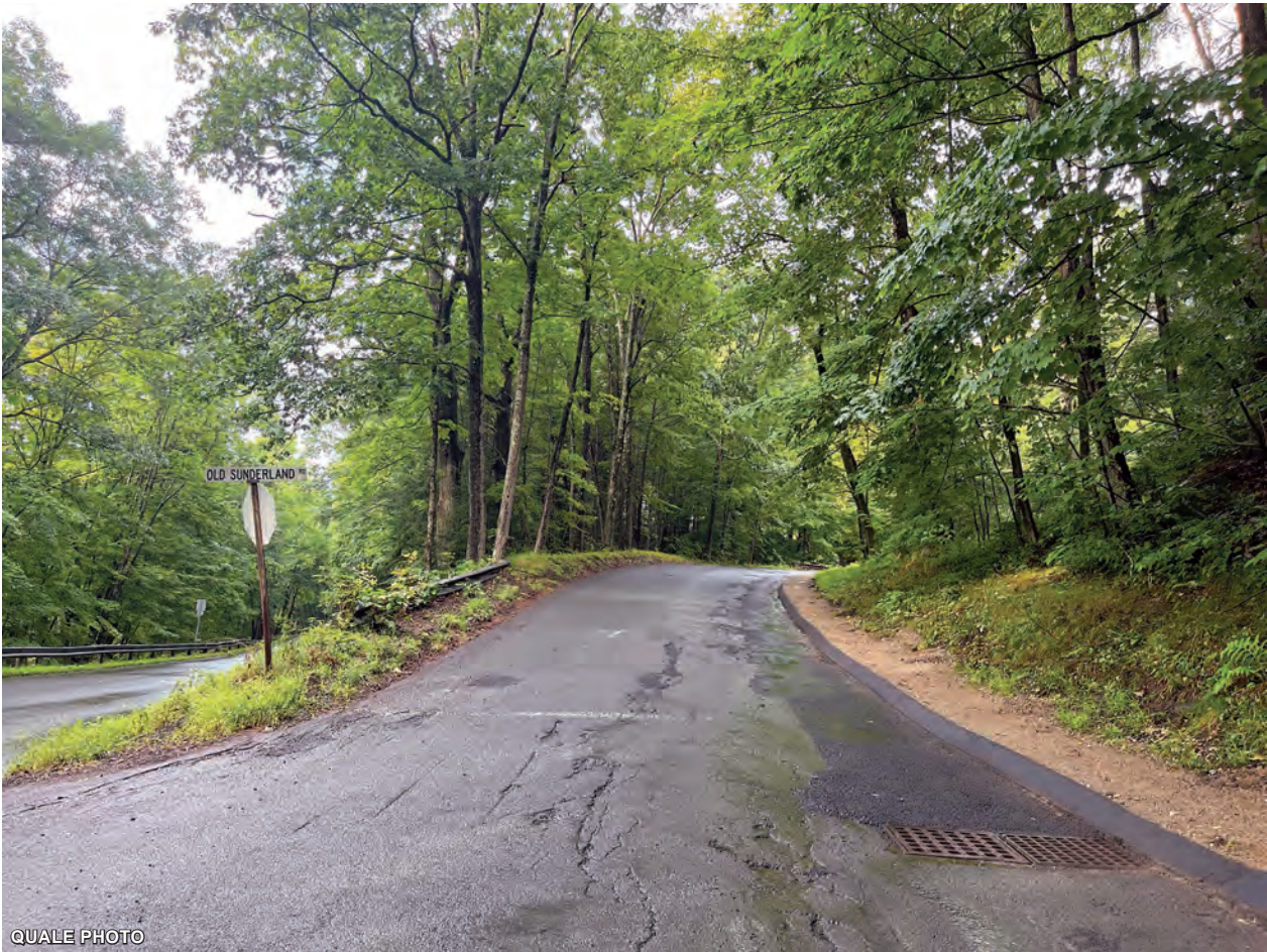
The DPW says it installed a new curb on Old Sunderland Road to contain runoff from a newly-widened driveway on the farm.
