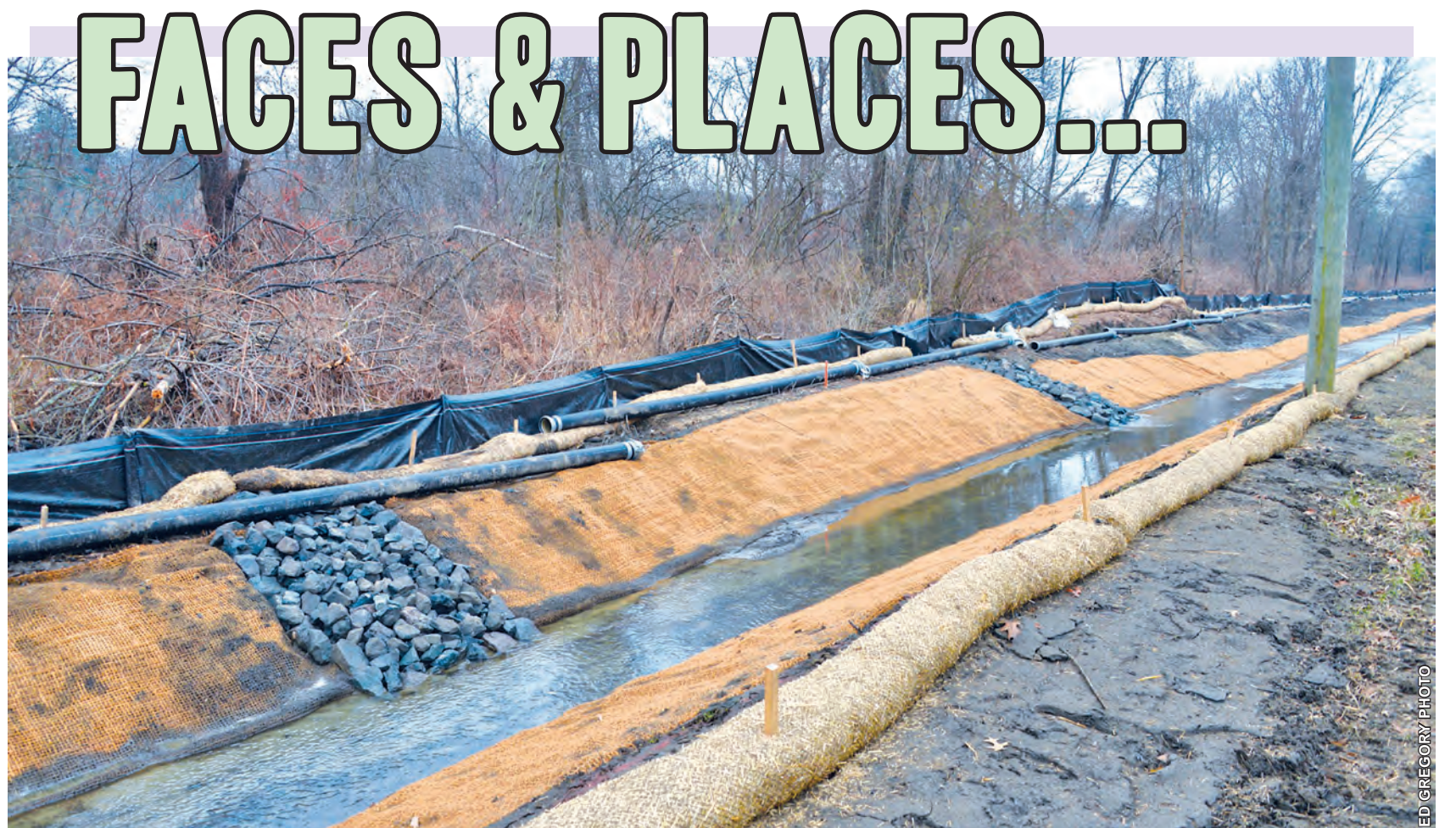
"The flood mitigation project currently underway along the east side of Montague City Road stretches for about 150 yards north-south, and is nearly halfway complete," writes Ed Gregory, who took the above photograph Sunday morning. "This should remediate the nagging road-soaking problem that has plagued travelers in past times."
