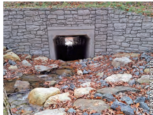
Third time's the charm: This culvert under Mormon Hollow Road is hoped to hold.
