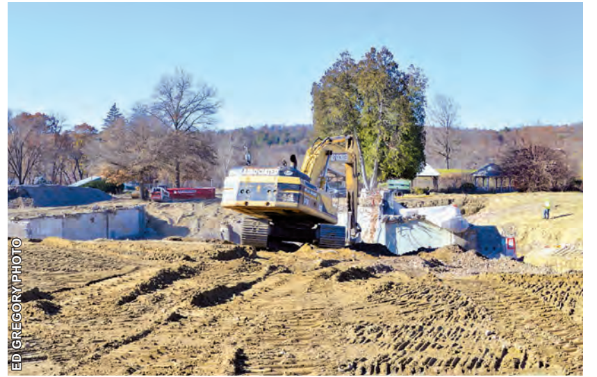
The view of the Farren Care Center property, from what had been the main entrance, on November 20. “The cleanup work will continue into December with final filling, grading, seeding and property transfer(s) taking place,” Ed Gregory reports.
