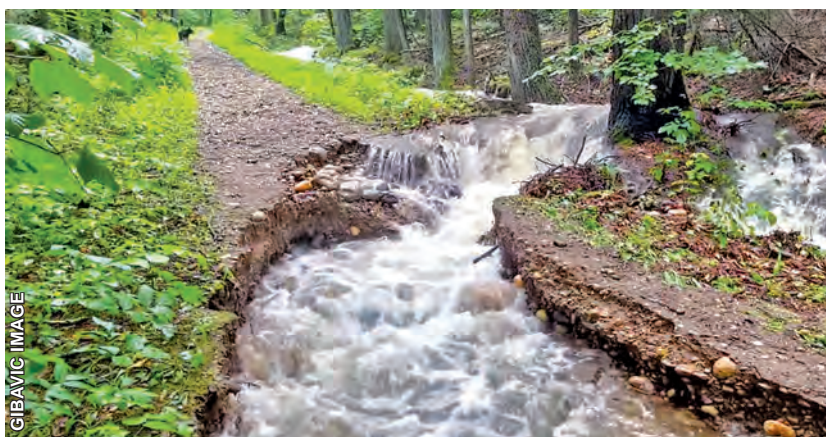
Video clips taken by Eva Gibavic during the mid-July rains show in vivid detail the damage they caused to the 19th-century road.
