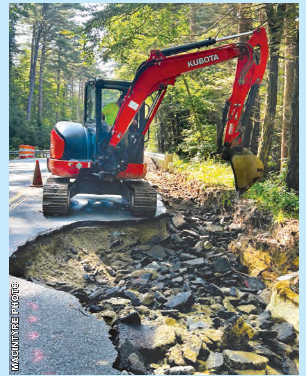
The microburst undermined two Wendell roads.
