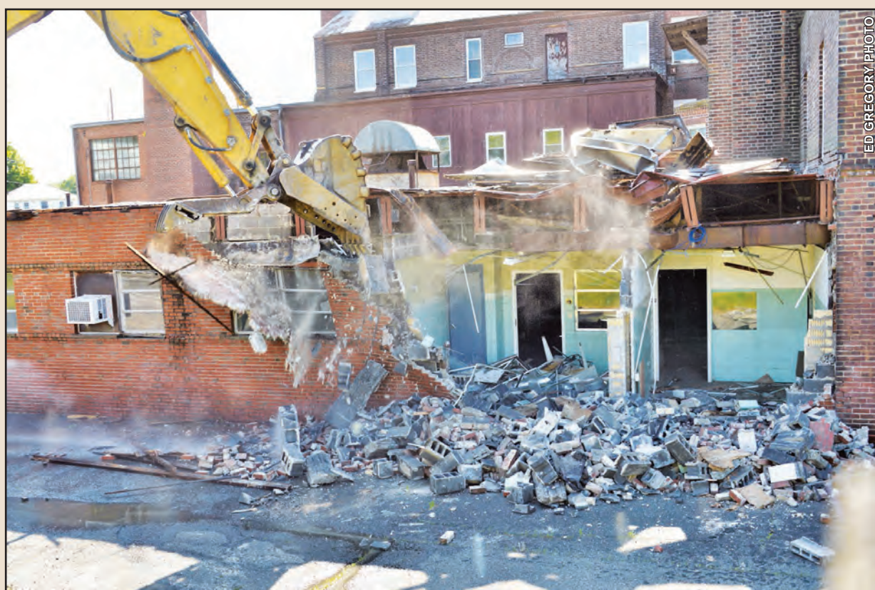
Demolition of the Farren Memorial Hospital in Montague City is well underway. "Associated Building Wreckers of Springfield, MA are charged with the razing project, which may take as long as a month to complete," Ed Gregory reported with this May 30 photo. "This photo shows the smaller of two excavators (Caterpillar 330D) taking a chomp out of the west side of the kitchen area wall, exposing the innards." This week the Montague Reporter reviewed video of the work taken by neighbors who say they believe the contractors are not taking sufficient measures to suppress dust. We are watching the story with interest.
