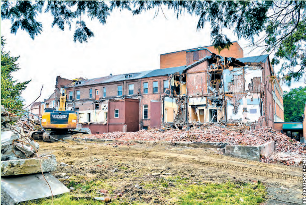
"The demolition project is about one-fifth of the way complete," photo correspondent Ed Gregory reports. "It's expected to go well into July, and possibly to August. The property reclamation will follow into September." This photograph, taken on Monday, shows the complex's west side, not visible from Montague City Road. Gregory describes it, left to right: "A section of the 1958 wing up to the brick elbow projection on the roof. The mid-area is a section of the 1960 wing, and the right side – the multi-colored wall to the end – is the 1928 wing. In the rear, the 65-foot high Farren Care Center building rises above the rubble."
