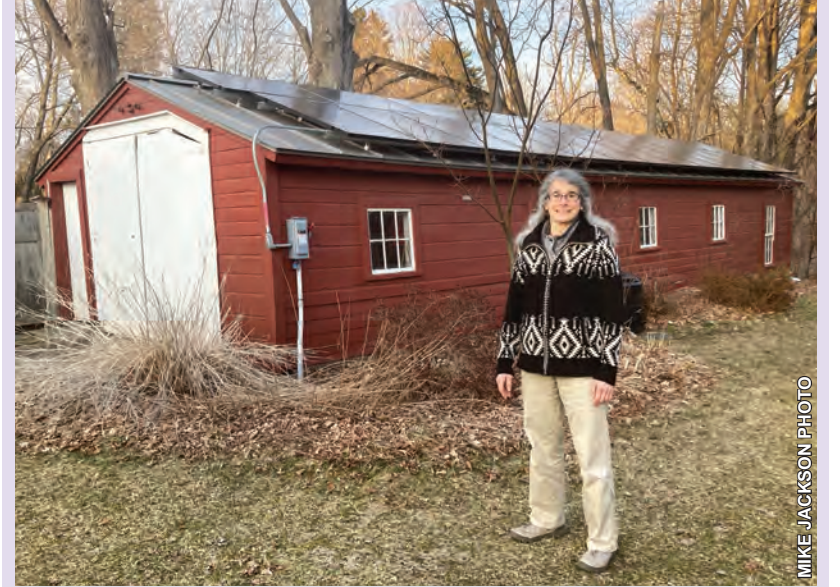
Energy committee chair Sally Pick says that four years after installing this 7-kW array on a small barn in her Montague Center backyard, she is running a credit on her electricity bill. Pick recommends homeowners interested in adding solar now pursue renewable energy certificates (RECs), as well as state and federal tax credits.
