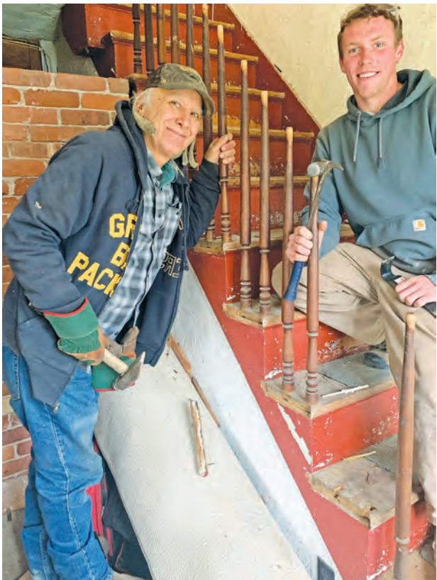
Dennis Lombardi and Ricky Smith, another local contractor who helped with the salvage, work the balusters out of the staircase.
