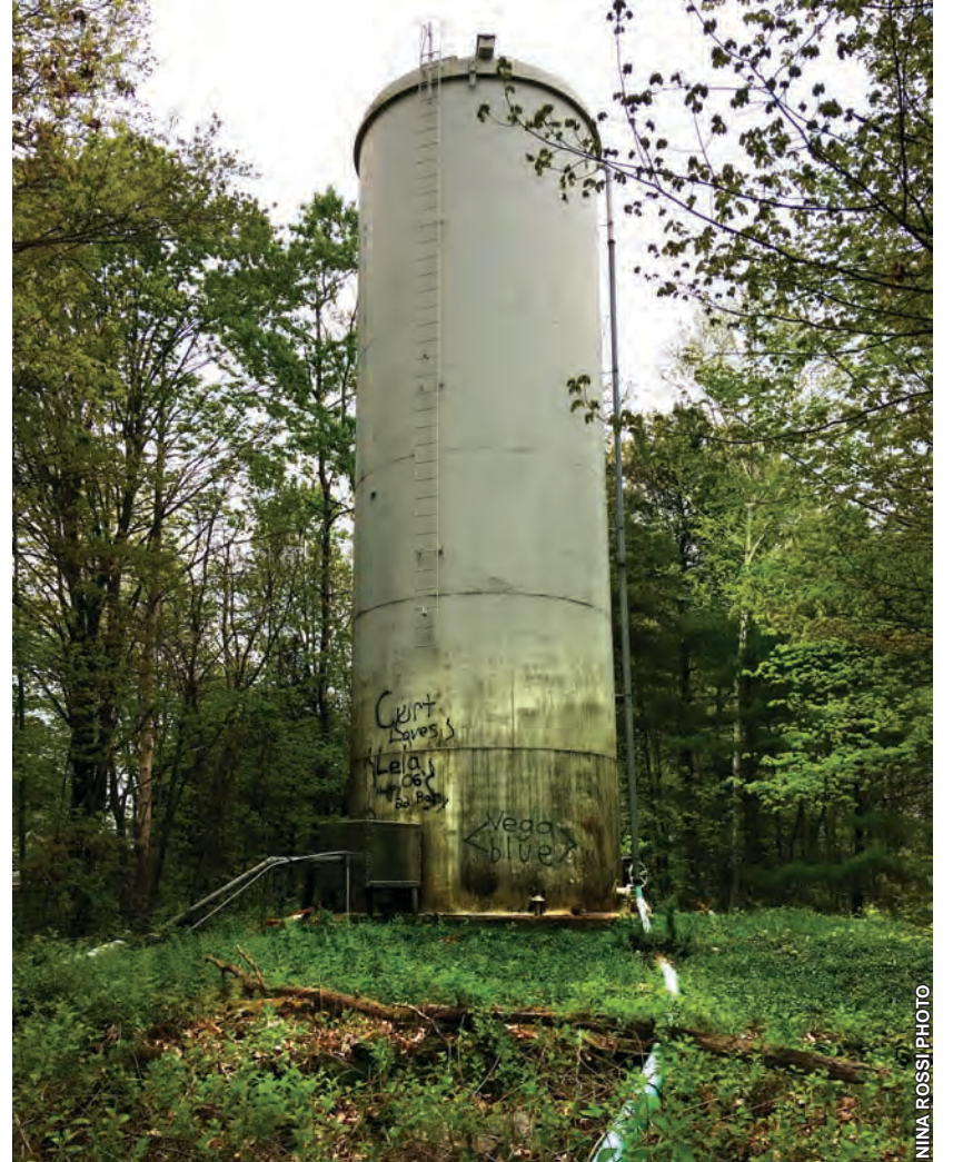
The district's water storage tank is in need of $150,000 worth of repairs. Some neighborhood residents are asking about a merger with the Turners Falls district.
