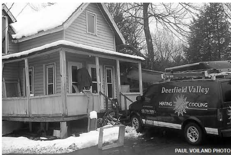
Deerfield Valley Heating and Cooling installed a free Lennox fuel efficient furnace for the Montague Energy Committee's raffle winner George Shapiro at his Lake Pleasant home last winter.
