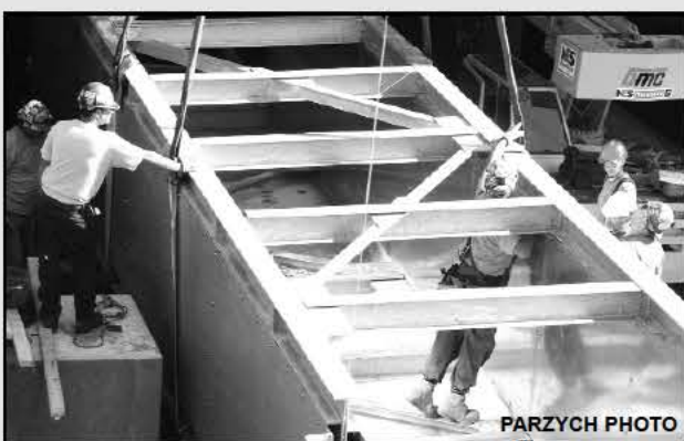
Last week, a shad-friendly galvanized steel box is lowered into place for improved passage beneath the Gill-Montague bridge
