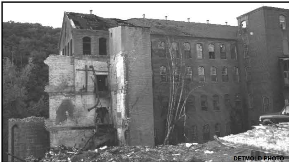
Building #1 at the Strathmore Mill, showing gaping holes in the roofline, following the May 26th fire. The town is in the process of taking the mill for back taxes.
