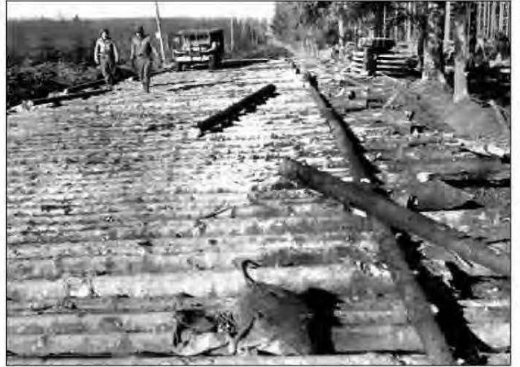
300th Engineers building a corduroy road of logs in the mud in Belgium.
