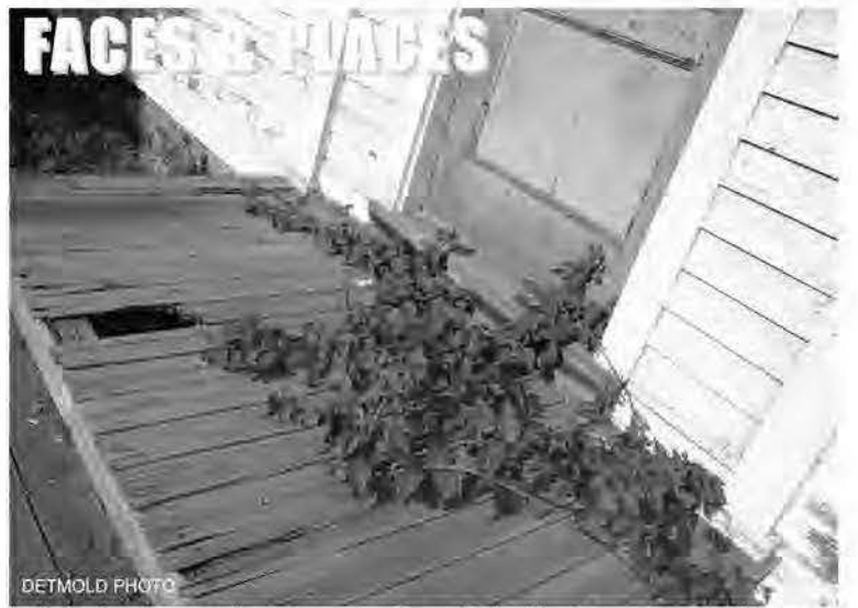
Woody nightshade presses up through the floor boards on L Street.
