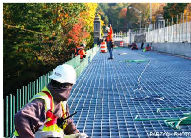
Earlier this week, workers readied a section of the Gill-Montague Bridge for concrete, laying the bridge deck grid onto stringers and tying into re-inforcing bars at left
