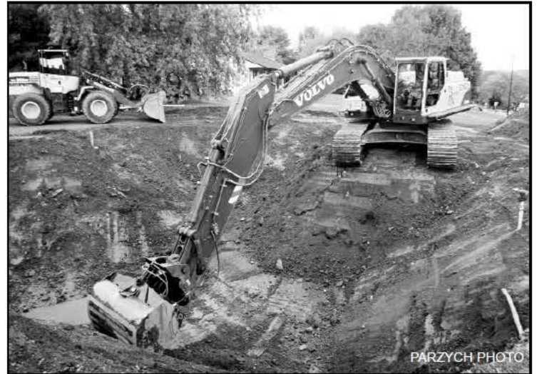
Dan Lively at the controls of Davenport's Volvo excavator digs deep for a new 12,000 gallon fiberglass reinforced double walled gasoline tank. Ground water is pumped out, filtered and sent down the sewer.
