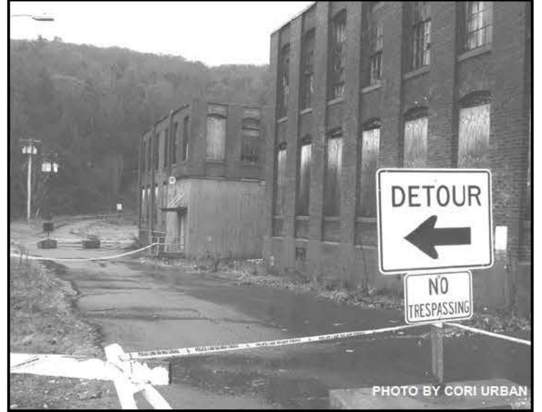
The roof of Building #1 (foreground) at the Usher Mill on Arch Street in Erving Center has collapsed.
