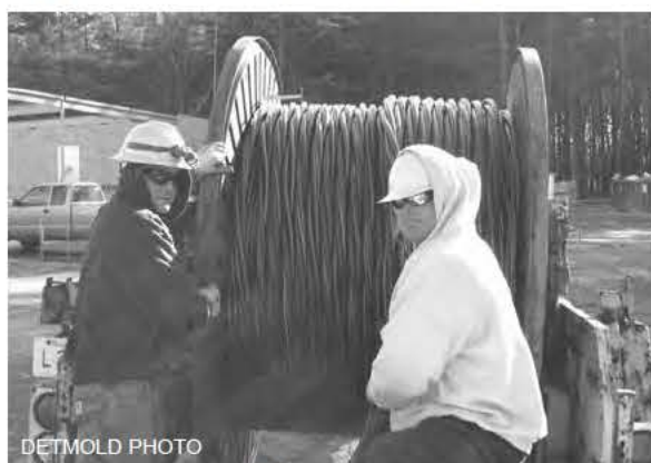
DETMOLD PHOTO Bill Freeman (left) and Tim Carlisle pull wire through an underground conduit to connect the new police station to the new utility pole on Turnpike Road
