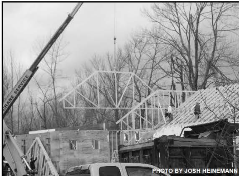
A crane lifts one of the library roof trusses into place on Friday, November 17th.
