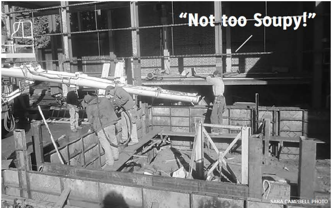
MONTAGUE CITY - On Wednesday, Valley Concrete from Bernardston, with the assistance of Lane Construction of Northfield, poured concrete for the foundation walls of the new garage at the Montague wastewater treatment plant. The extension of the operations building will make room for a new Fournier rotary dewatering press to reduce the volume – and the cost – of sludge hauling from the plant.
