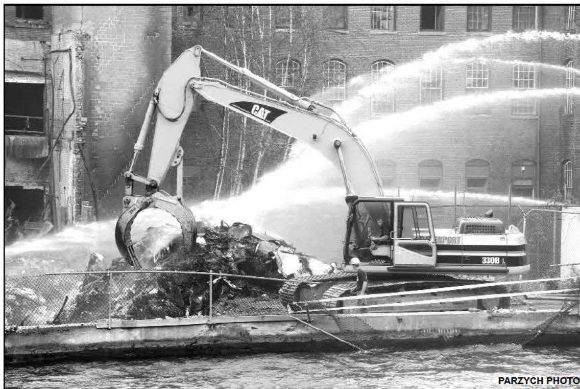
Davenport Construction's excavator digging up smoldering debris on Sunday at the Strathmore while firefighters hose down the hot spots.
