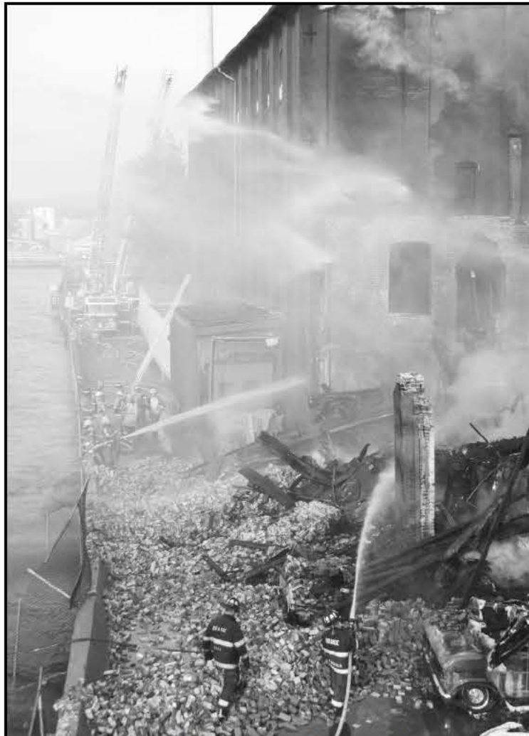
This photo, taken Saturday at approximately 7 a.m., shows Turners Falls Engine 2 and the Turners Falls ladder truck backed up by the Northfield ladder truck pouring water on the blaze while Greenfield's pumper adds more water power from the bike path across the canal.
