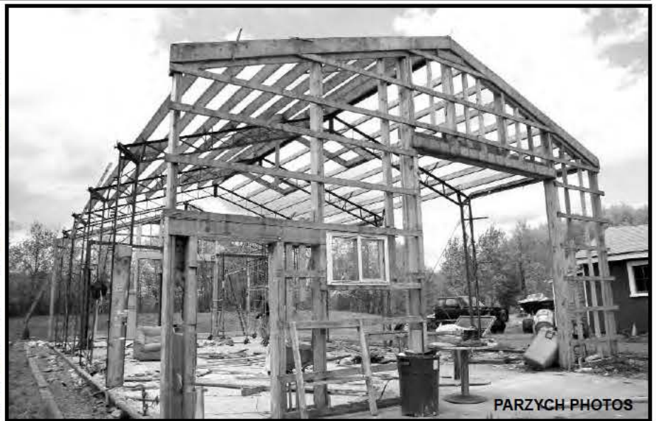
Rusty Coombs dismantling Koch barn in Turners Falls to resurrect in Colrain.
