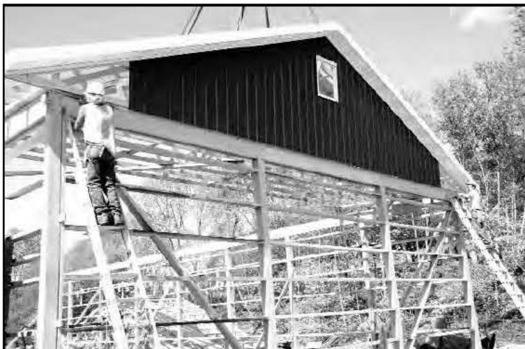
The gable end of the roof has siding installed prior to hoisting into place.
