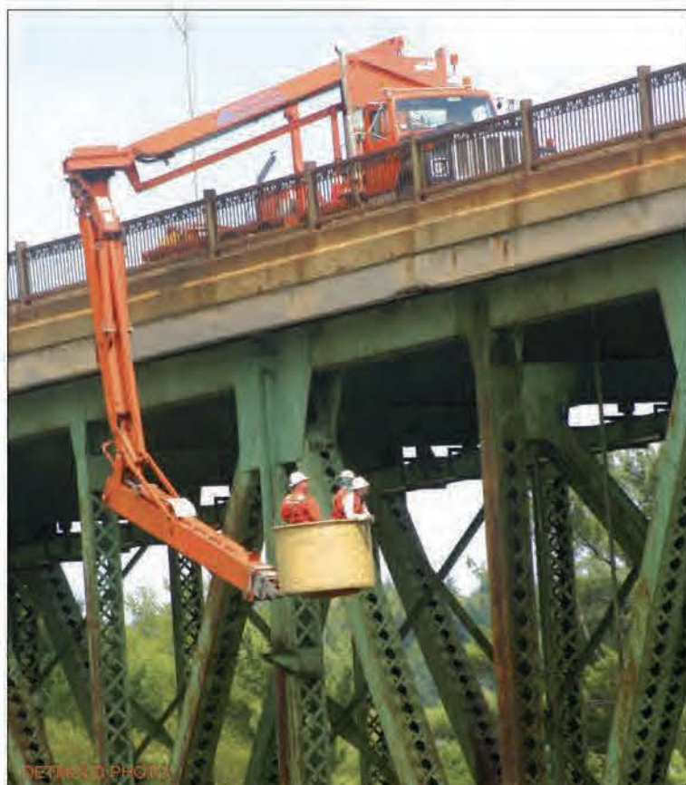
Two engineers from HNTB Corp. (right), with a MassHighway employee at the extension arm controls, inspect the girders of the Gill - Montague bridge on Tuesday.
