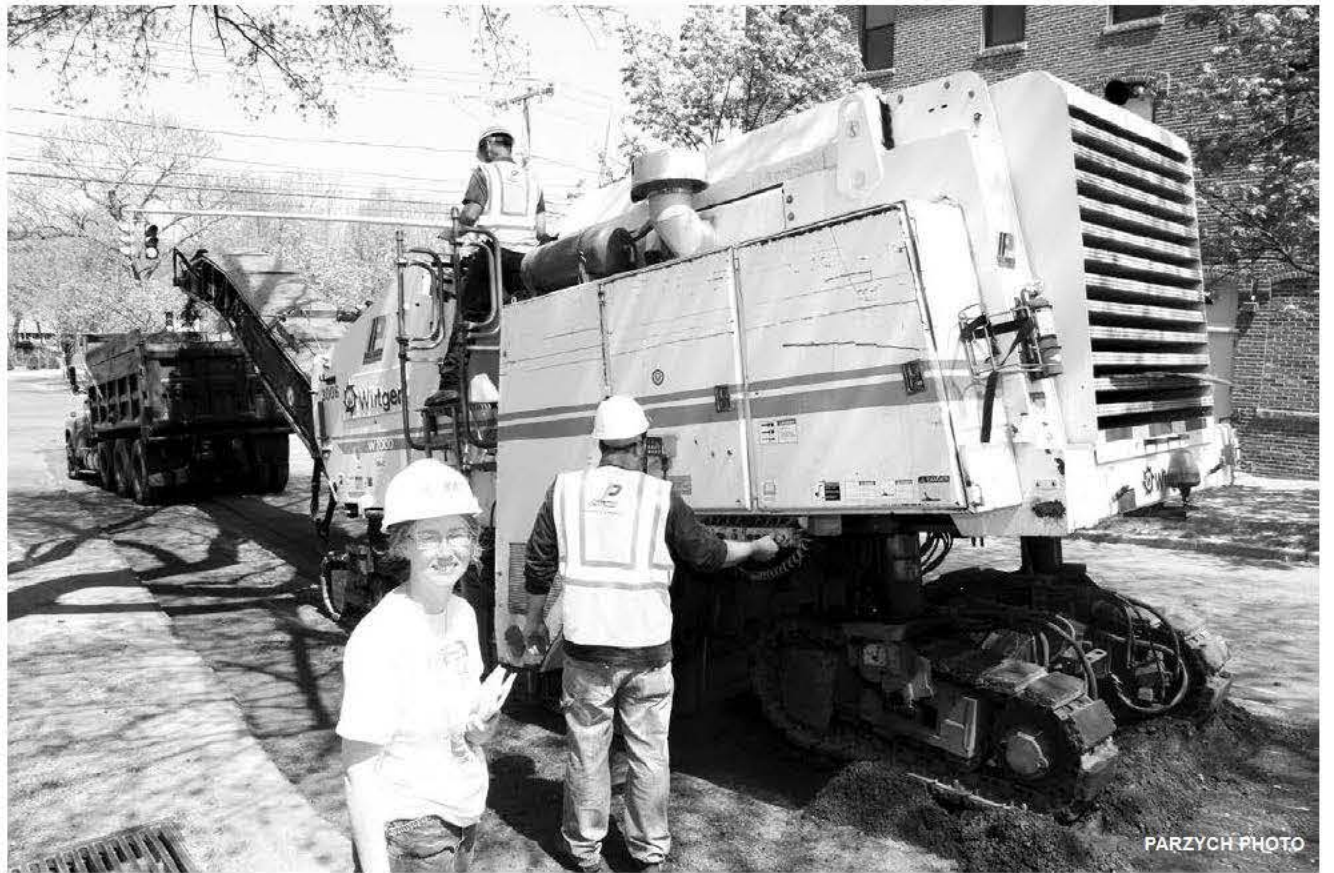
Engineer Sara Campbell keeps watch over pavement removal by the Carnegie Library on Wednesday. She reports that the 7th Street trench shows no signs of settling, and was solid when the roller passed over it.
