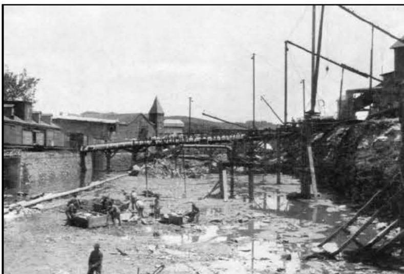
Early 1904: Excavation of the Power Canal. Photo by permission from Montague Labor and Leisure by Kyle Scott.
