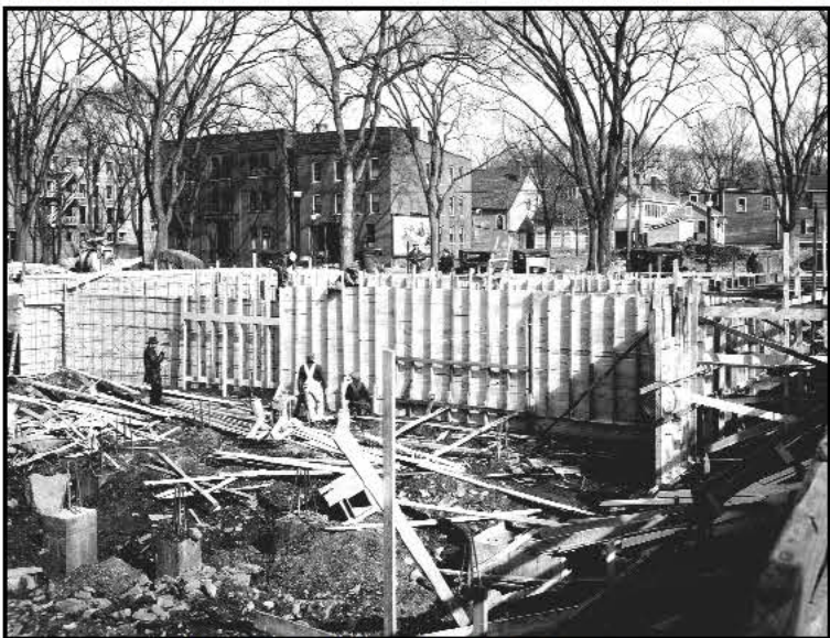
March 29th, 1935 - The front wall is formed. Turners Falls Inn on the left.
