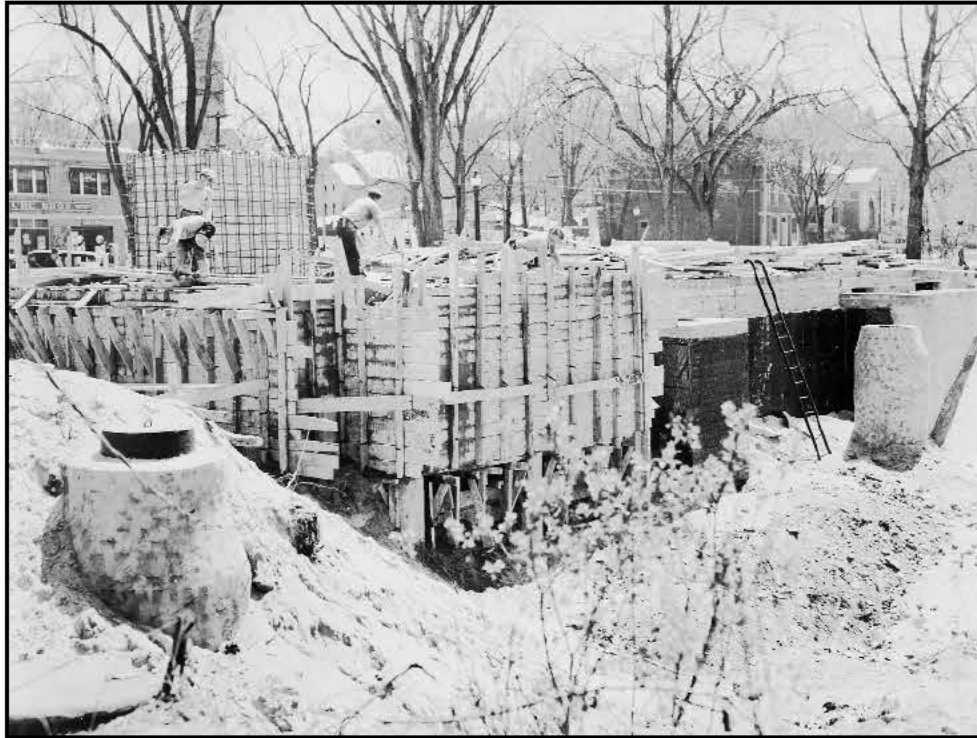
In this photo, the photographer was facing southeast. Couture Bros Gas Station can be seen at left; St Kazimierz and Carnegie Library at right. Foundation walls with manhole in foreground.
