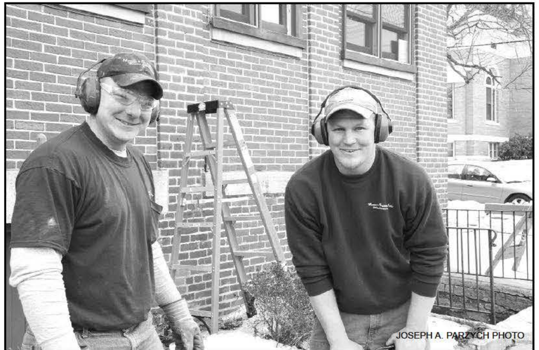
Morny & Schmidt employees Seth Hagar and Mark Peterson work on breaking up sidewalk for pier footings for a new smoking deck for St. Kazimierz Hall on Avenue A in Turners Falls. Hagar and Peterson happen to be smokers, and seem satisfied with the assignment.
