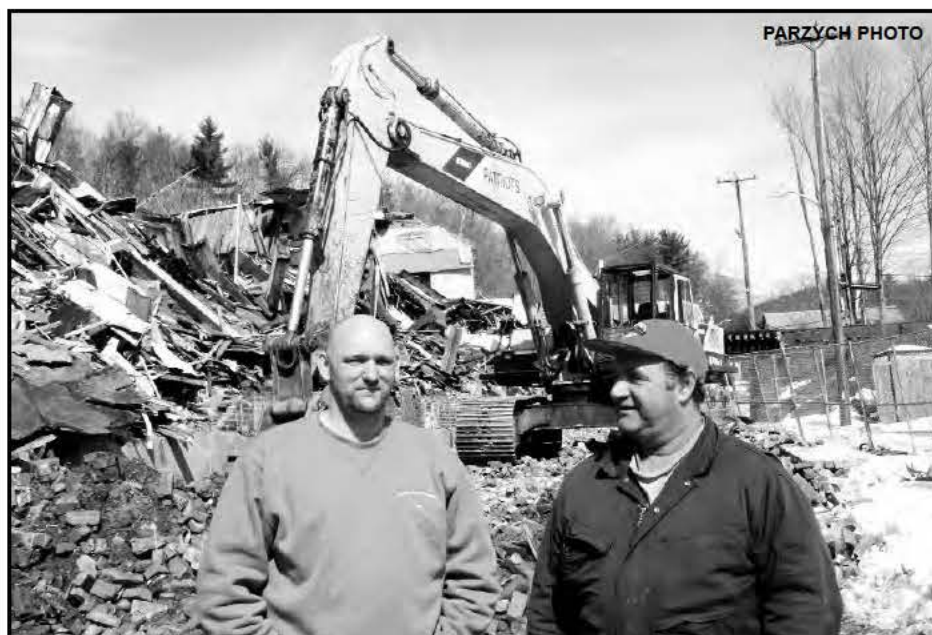
Kurt Bussiere, left, who co-owns the Patriots Environmental Corporation of Worcester, stands with excavator operator Gary Bond in front of the former Usher Mill in Erving.
