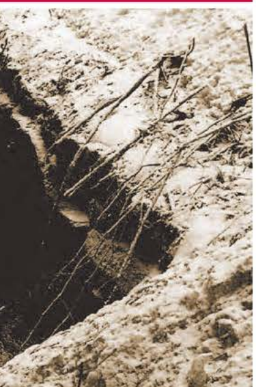
Water backed up at the culvert on Bull Hill Road on Monday
