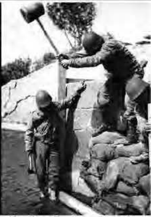
300th Combat Engineer Battalion repairing the under piling of a bridge destroyed by enemy fire along the Carentan - Cherbourg Road in France - June 30, 1944.
