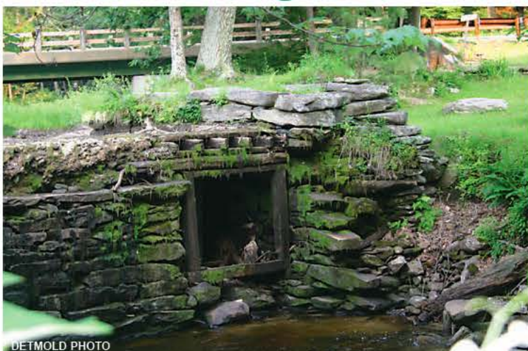
The square opening in the North Leverett dam once held a power wheel for a blacksmith shop on the south bank of the Sawmill. Last week, this side of the dam was breached after heavy rains, and is now in need of emergency repair.
