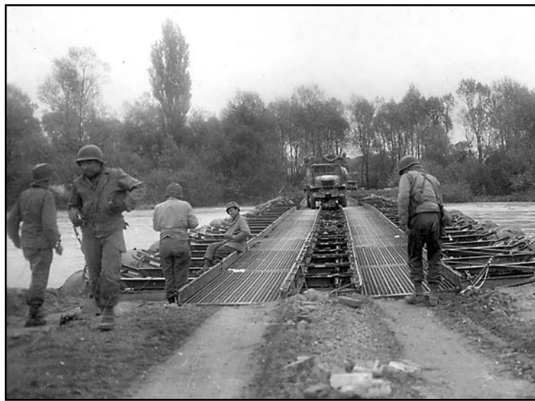
The 300th preparing to build a bridge over the Isar River beginning April 30th and finished in early May 1945.
