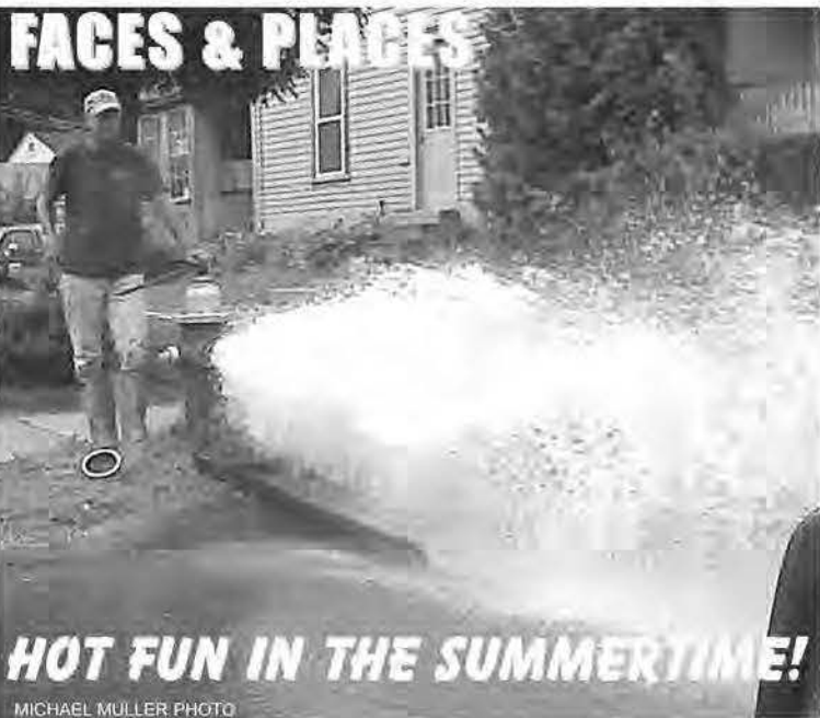
John Collins of the Turners Falls Water Department flushing a hydrant on L. Street on Tuesday.
