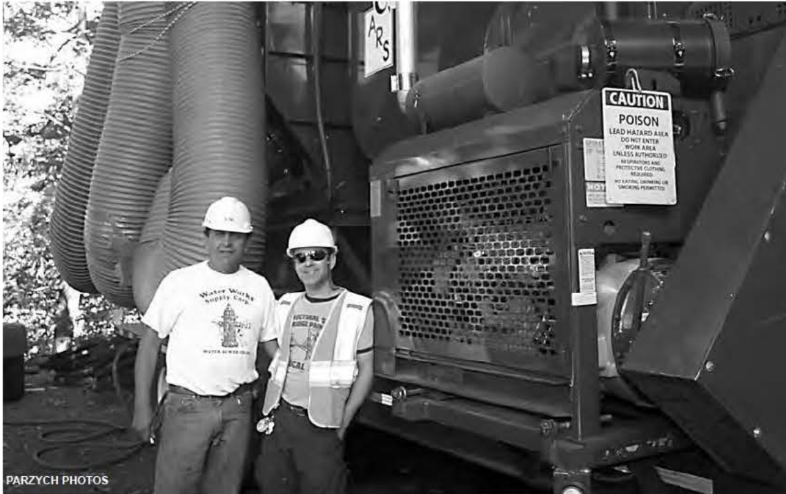
John Tiliakos, left, and his fellow Mimosa Construction supervisor, Nikos Kantzoglou stand in front of the dust collecting machinery and air ducts connecting the collector to the canvas covered underbelly of the G-M Bridge.
