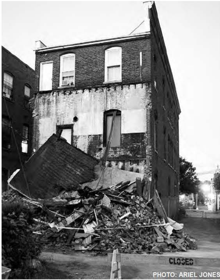
This two-story brick wall in the rear of 62 Avenue A came crashing down Sunday night, leaving tenants to scramble for shelter in the middle of the night. No one was injured.
