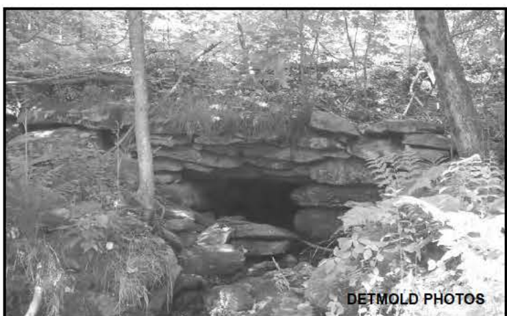
One of the few remaining culverts that once kept spring rains from washing out Dry Hill Road.
