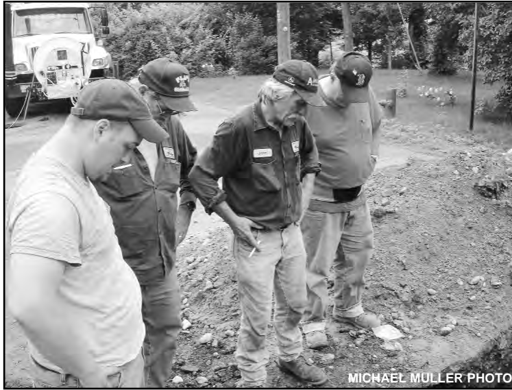
A crew from the Montague DPW examine the 10-foot sinkhole that appeared in the middle of Center Street earlier this week.
