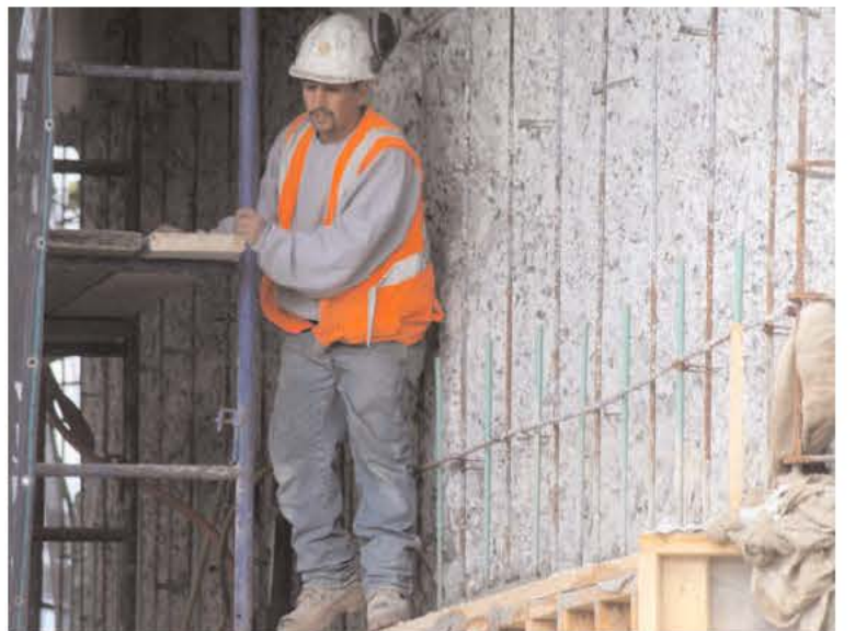
An SPS carpenter works on forming exposed reinforcing rods on the bridge abutment on the Turners side of the bridge.
