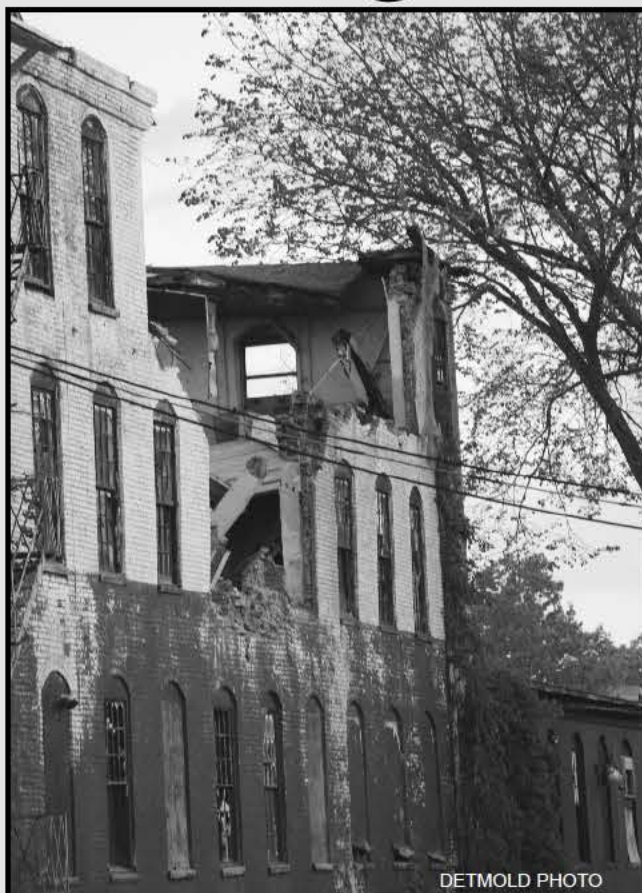
Part of the northwest wall of the Railroad Salvage building collapsed into Power Street on Saturday
