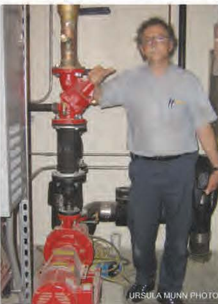
Building committee member Jason Burbank stands beside the geothermal well field pumping system at the new police station.
