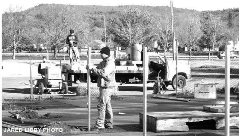
Dan LaValley and his L & L Fence crew install fencing at the Turners Skate Park on Tuesday
