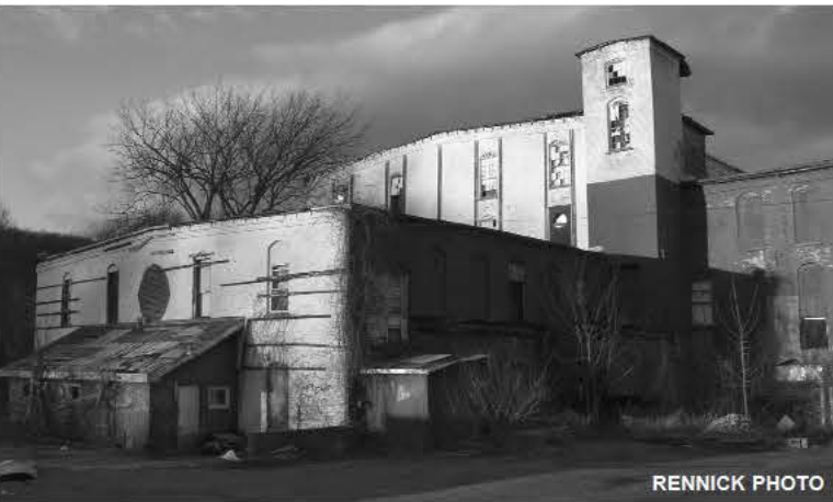
Sections of the roof of the Railroad Salvage building have collapsed into the basement.
