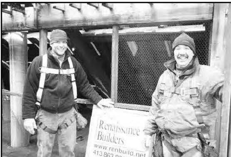
Bryan Grunwald, left, and Andy Stevens, right, lead carpenters on the Strathmore Roof repair.
