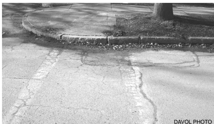
This Avenue A crosswalk has no curb cuts for wheelchair accessibility. Grant funds will pay for reconstruction of walks up and down the Avenue
