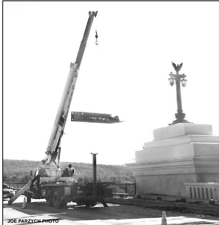
Springfield Steel Erector's crane lifts a steel pan filled with trap rock stone to lower to abutments beneath French King Bridge on Monday
