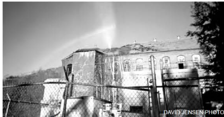
On Saturday, November 24th, when a sprinkler pipe in Building #1 froze and burst an elbow, it sent a geyser of water up through the burnt out roof, where it continued to spout in the early morning light like a beached whale.
