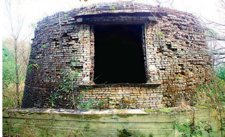
With weeds and small trees sprouting from the roof and bricks falling, the kiln still stands after more than a century, defying heavy snow loads and the forces of gravity.
